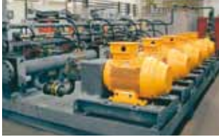
Pump station for strip-winding plant
