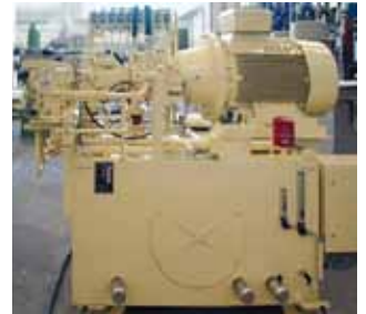
Bucket wheel excavator: Hydraulic power unit
