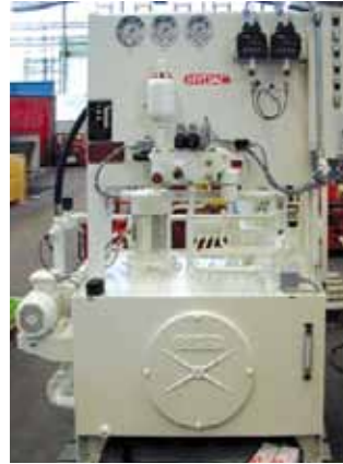
Cement mill: Hydraulic power unit
