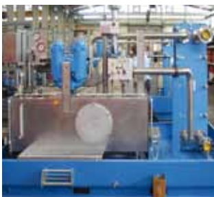
Refinery: Hydraulic equipment
