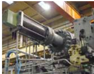
Slam-shut valve to protect against turbine overspeed
