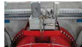
Hydroelectric power plant: Power unit for gravity actuated butterfly valve in cooling water circuit
