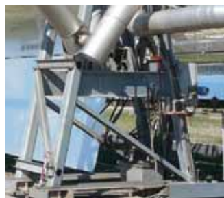
Solar thermal power plant: Power unit for parabolic reflector adjustment
