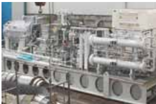
Oil system of compressor plant
