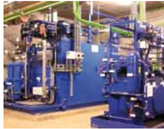
Control oil supply for steam turbine
